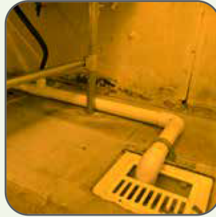
Figure 7: Piped drainage running into floor sink
